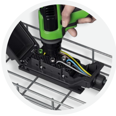
Copper displacement connection of the cable
